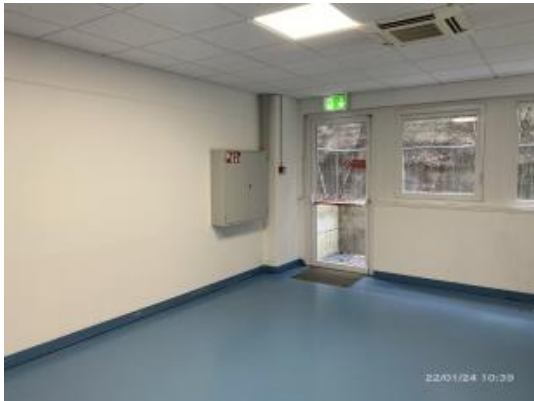
Emergency exit - Fire fighting equipment - Fire alarm system.JPG
