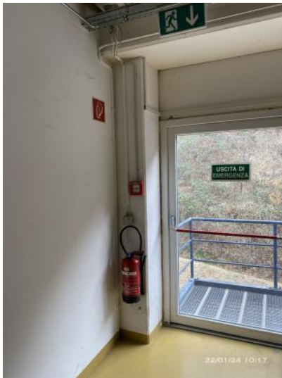
Emergency exit - Fire extinguisher - Fire alarm system.JPG
